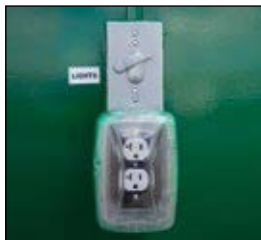
Weatherproof GFI receptacle and light switch
